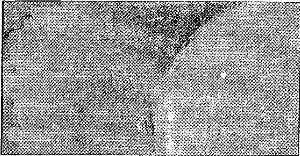
Br #9340 I-35W Over Mississippi River Typical Weld Cracks on Top Web/Flange Weld And Top Vertical Stiffener/Web Girder
